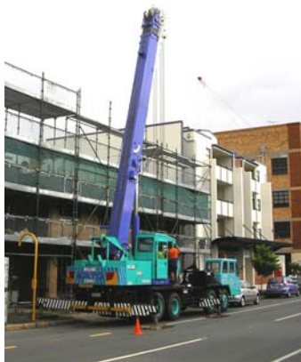
Figure 2 – Hazard striping on a mobile crane
